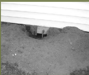
Damage from skunk burrowing
