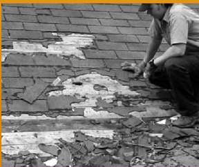
Roof damage from mother raccoon
