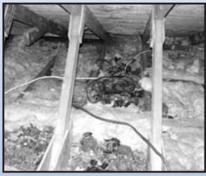
Contaminated insulation from raccoon
