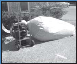
Vacuum removal system
