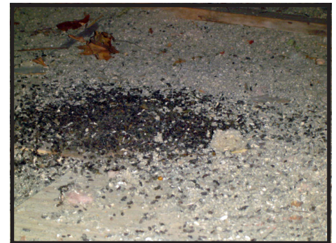
Insulation contaminated with bat guano
