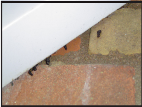
Bat entry point and droppings
