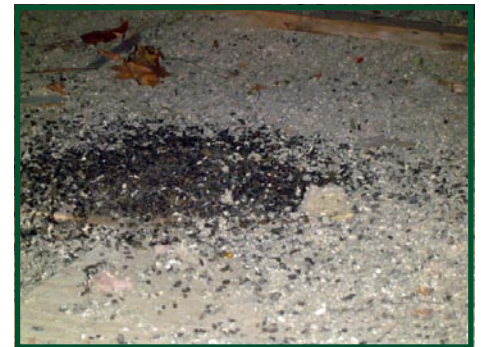
Insulation contaminated with bat guano
