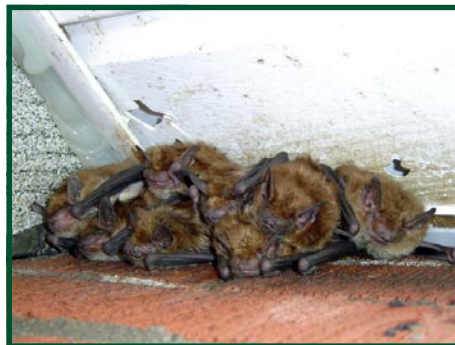
Bats roosting in corner of attic
